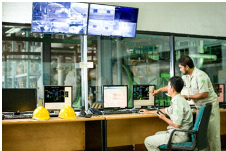
Gambar Distributed Control System (DCS) di Produksi
